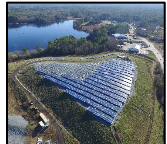
1.8 MW NORTH CAVER, MA
