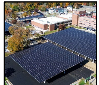
2.8 MW BROCKTON, MA
