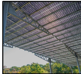
1.19 MW GLASTONBURY, CT
