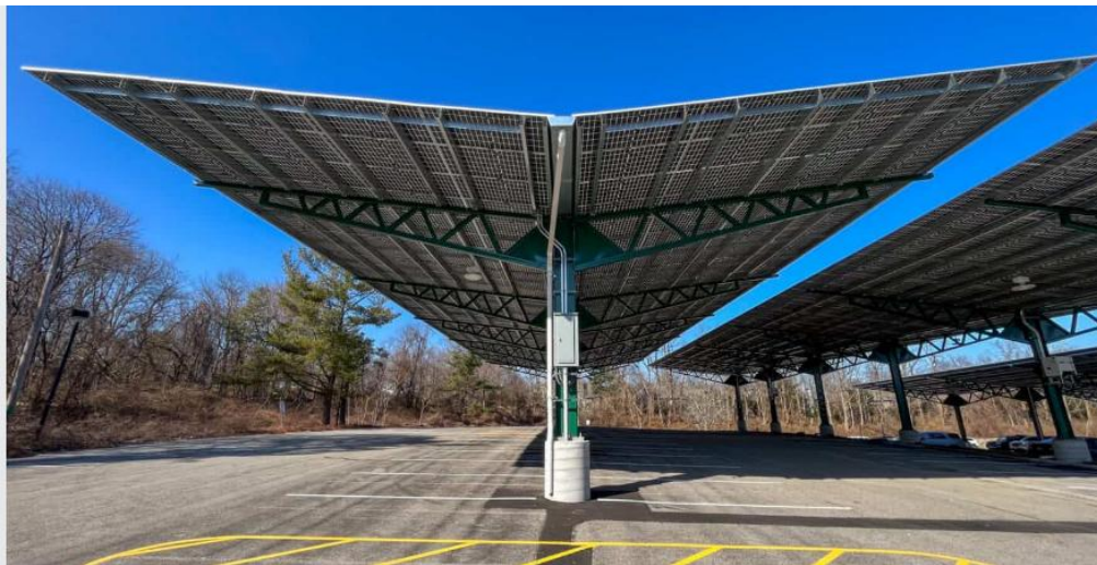
Figure 3. DC / AC Electrical Work Boxes Accessible by Authorized Persons
