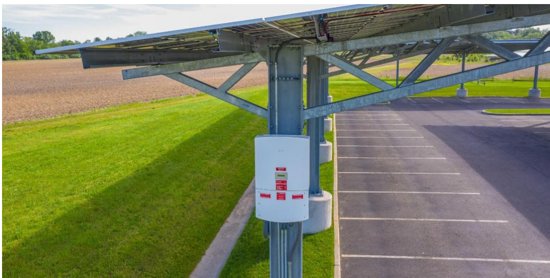
Figure 2. Inverter mounted away from the PV modules
