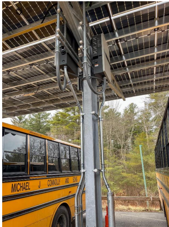
Figure 4: Unistrut supporting Inverters and Input / Output Conductors Outside the I-Beam
