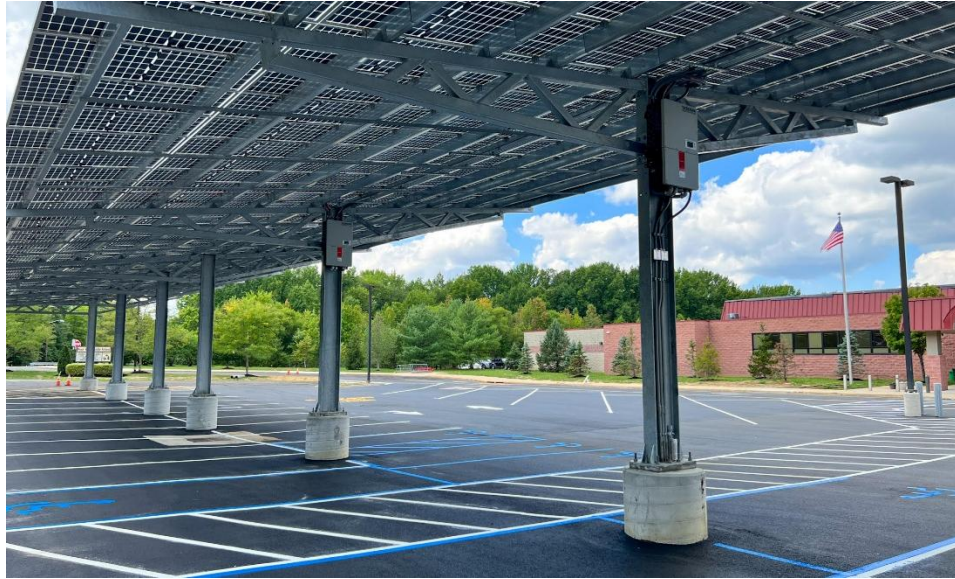
Figure 1. PV Grid Tie Inverter mounted near the top of the Solar Carport Post
